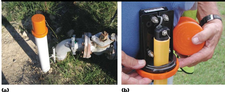
(a) Typical pipe protection RMUs installed to interrogate the pipeline and transmit system corrosion control effectiveness data. (b) RMU with cap removed showing terminal connection points.
